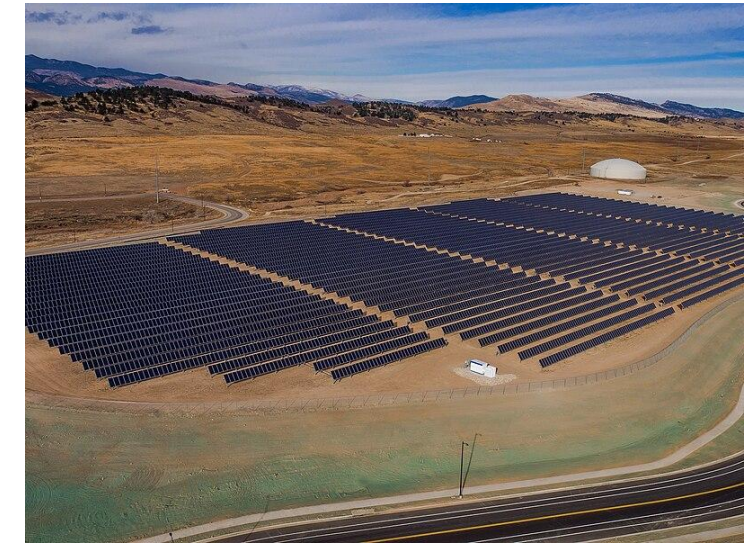
Solar Photovoltaic energy
